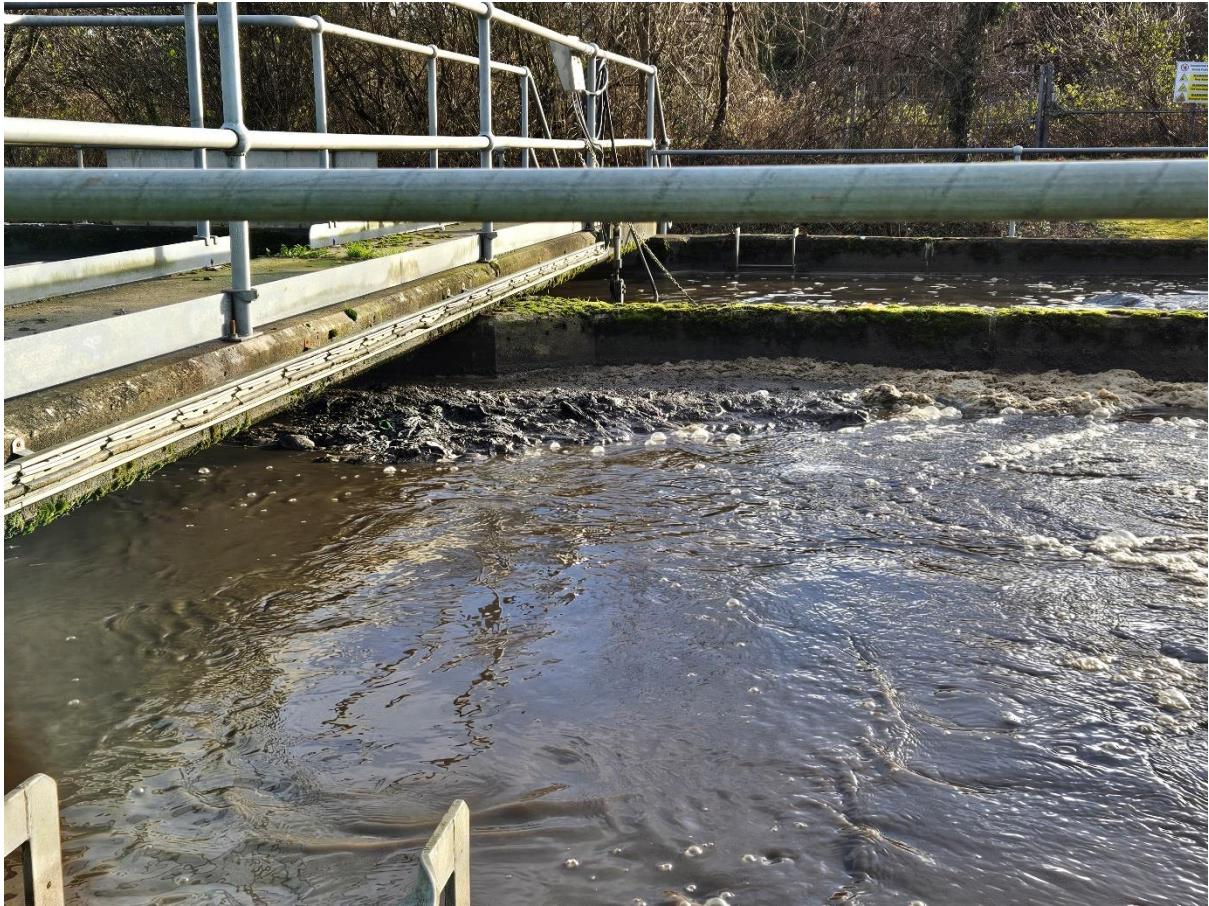
Photograph No. 2: Excessive build up of solids observed in both oxidation ditches affecting the effectiveness of treatment provided.
