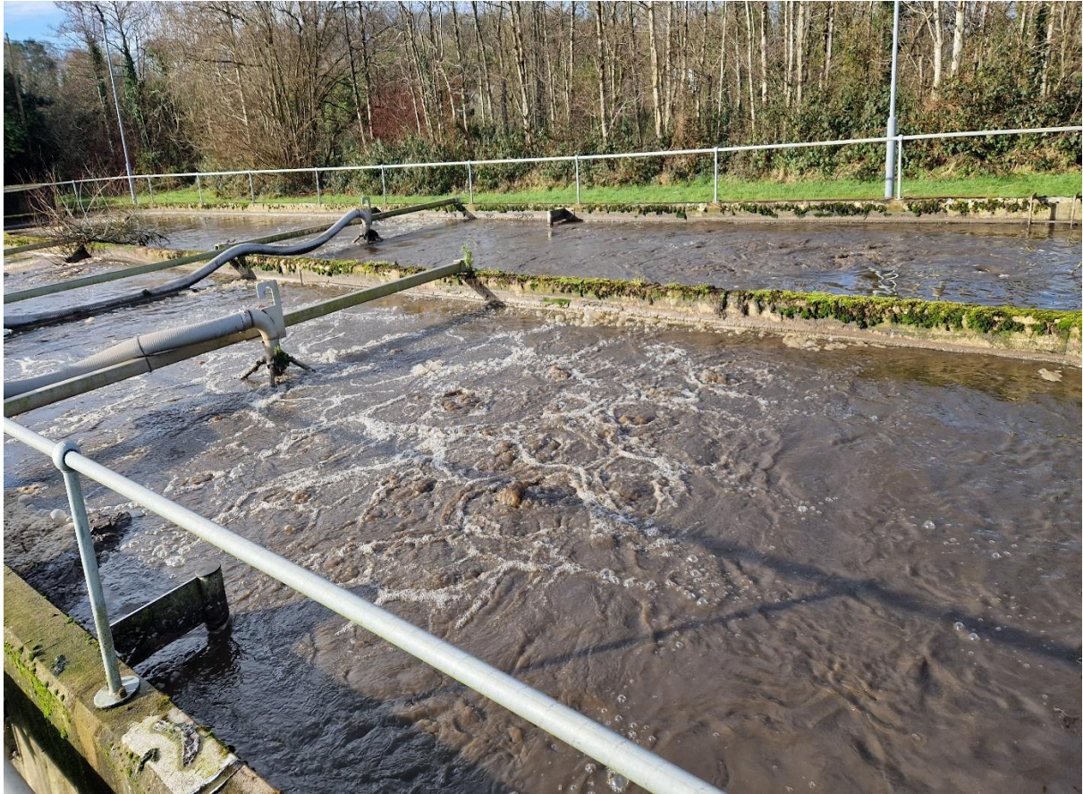
Photograph No. 1: Uneven distribution of air from the diffused aeration system due to multiple broken diffusers attributed to excessive ragging and build up of solids in both oxidation ditches.
