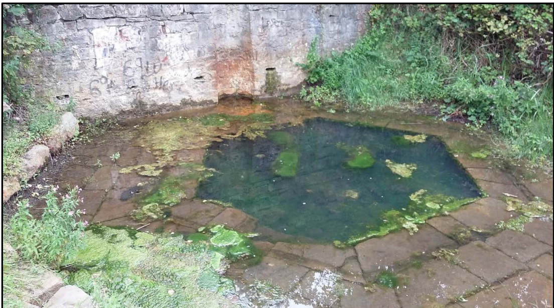
Photograph 4: Current condition of spa well and cistern (13 th August 2019)
