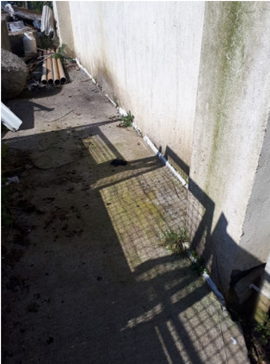
Photo 3: The walls of storage shed may not be water-tight. These storage shed walls need to retain firewater under the current firewater retention plan.
