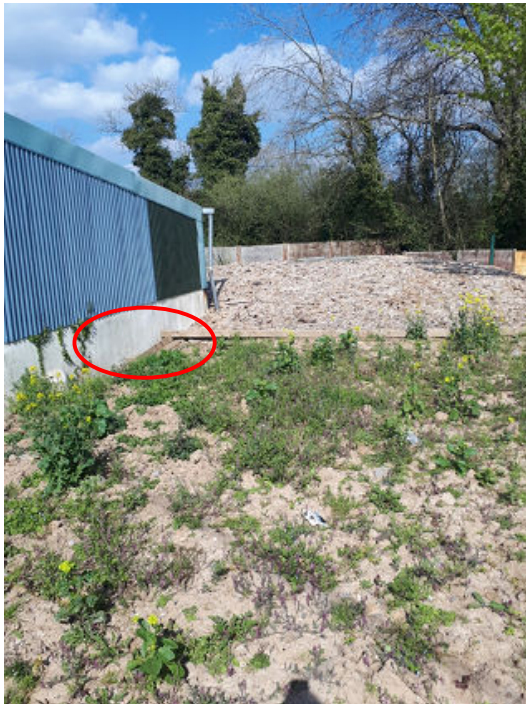
Photo 4: A number of large cracks were noted in the shed rear wall as indicated by the red circle
