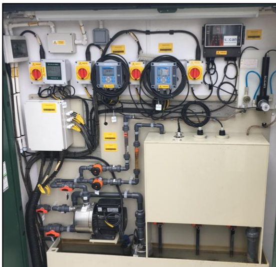
Figure 1 – Example monitoring sensors
