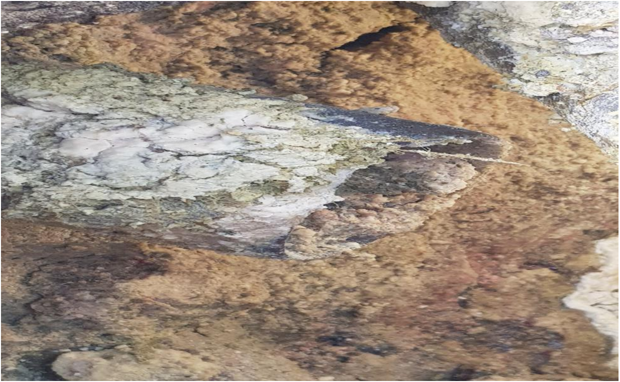
Photo 7: Photo taken in manhole (FM19) which is in very poor condition with an accumulation of congealed fat and solids in the foul pipelines leading to the WWTP.
