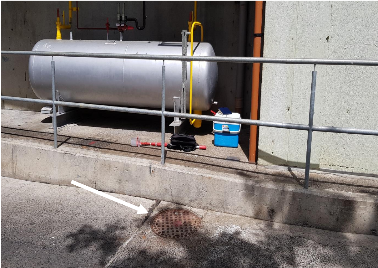
Photo 5: Manhole (Ref: F18) is located outside of the chilling rooms and boning halls (indicated by the white arrow). The unauthorised discharge pipeline at the riverbank was traced back to this manhole by the licensee. This manhole is on the foul line which carries effluent and washings from this area to the WWTP.
