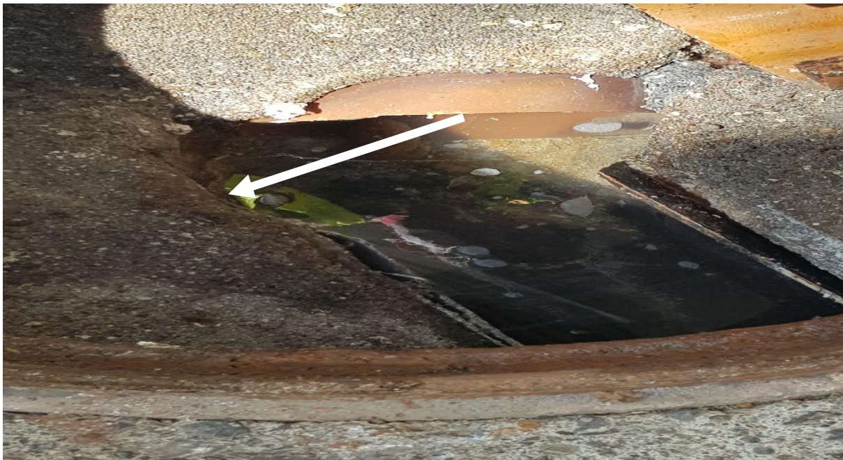
Photo 6: Photo taken inside the manhole (Ref: 18). The licensee considers that corrosion to the concrete within the manhole (indicated by the white arrow) permitted an unauthorised discharge of effluent and washings to the River Nenagh on 02/07/2019.
