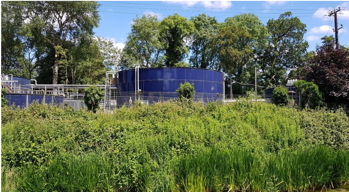
Photo 1: Waste water treatment plant (WWTP) at ABP Nenagh (taken from across the river).
