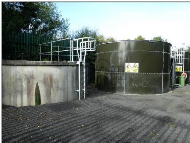
Plate 7 The Ballyclogh WwTP.
