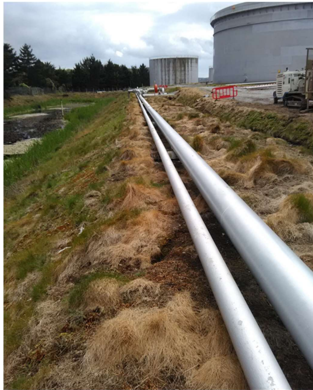
Image 9. View west along the oil pipe rack on northern side of the existing Catchment Basin CB1.
