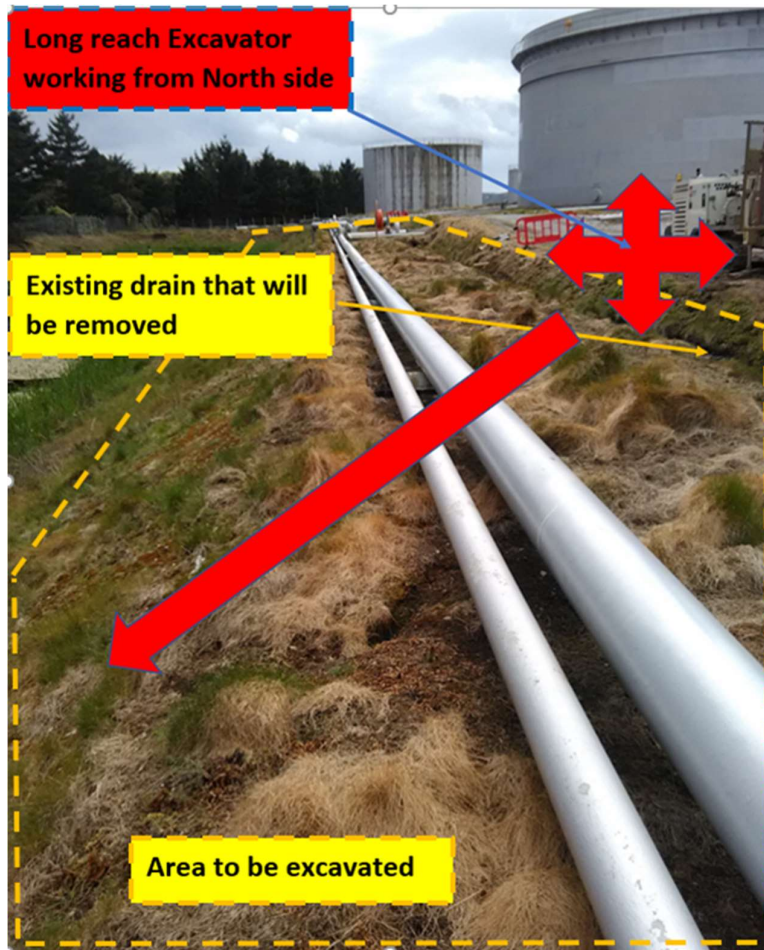
Image 11. It is envisaged that works will be carried out from the Northern side using a long reach excavator, periodically reversing the bucket to get access under the existing pipe work. The existing drainage channel will be removed by the works and temporary measures will be required during construction. The existing pipework will need to be protected from accidental damage throughout.
