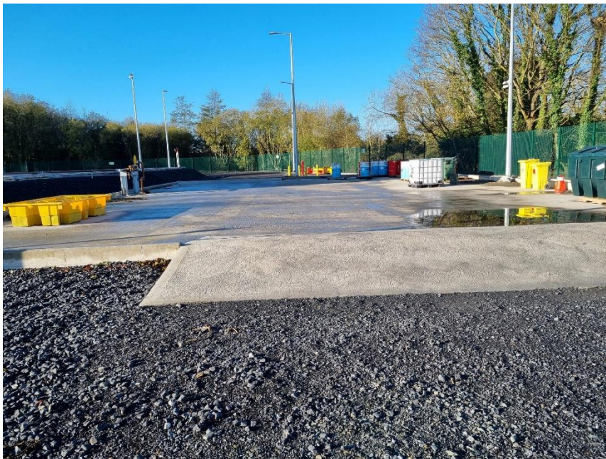
Picture 3: Fuel intake area and bund
