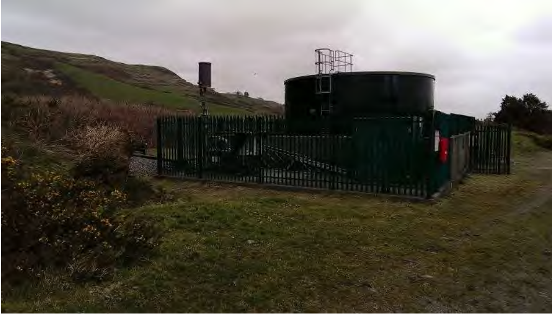
Photo 3.2 Leachate Collection Tank and Landfill Gas Flare
