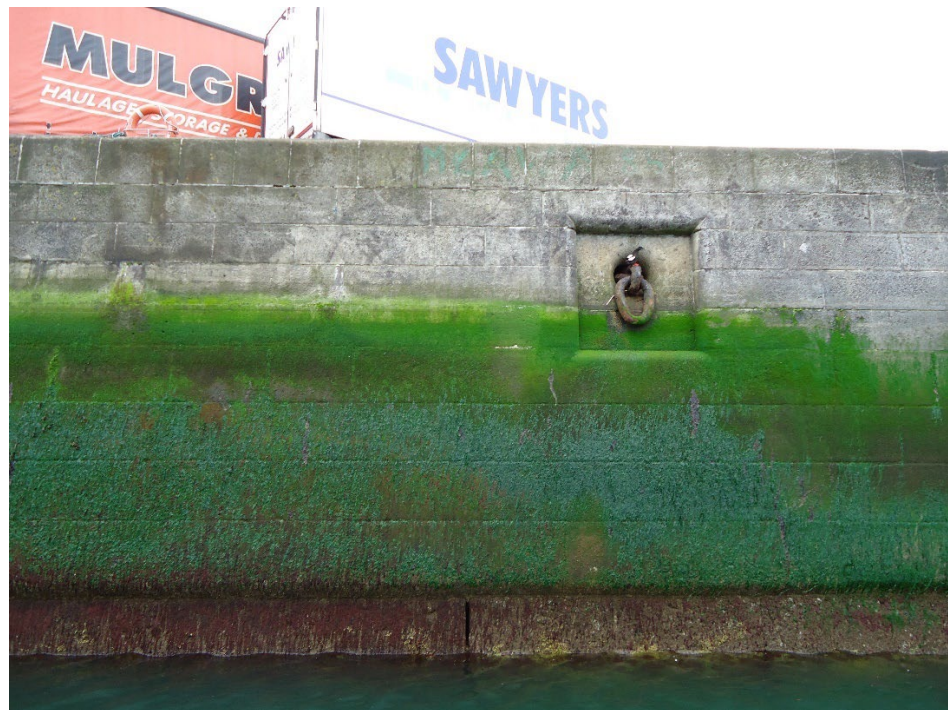
Photograph shows the top of two mass concrete foundation blocks and the join between both at the base of the image, with the granite ashlar coursing constructed above and a recessed mooring ring
