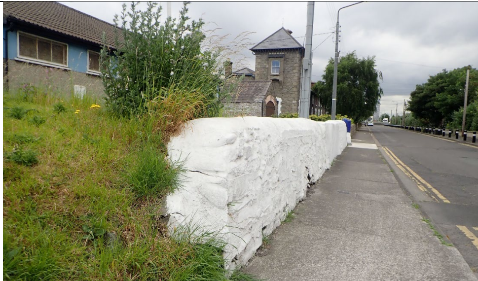
View looking west along Pigeon House Road, showing the southern parapet of the GSW as it survives serving as the boundary wall to the Ringsend Sea Scouts den
