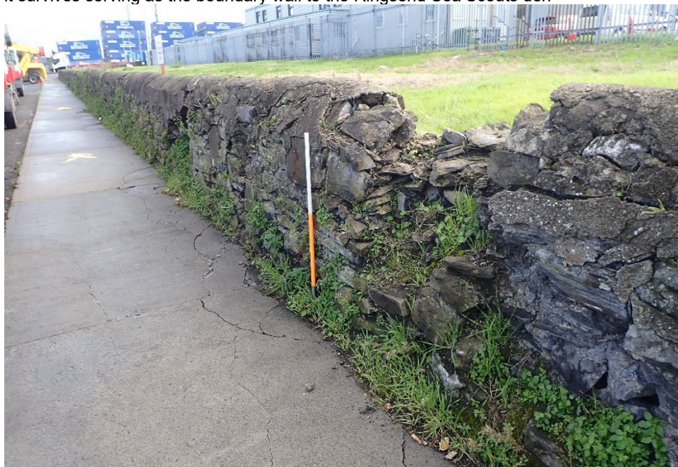
View looking east along upstanding southern parapet of the GSW that retains the north side of the grass verge in the MTL Yard
