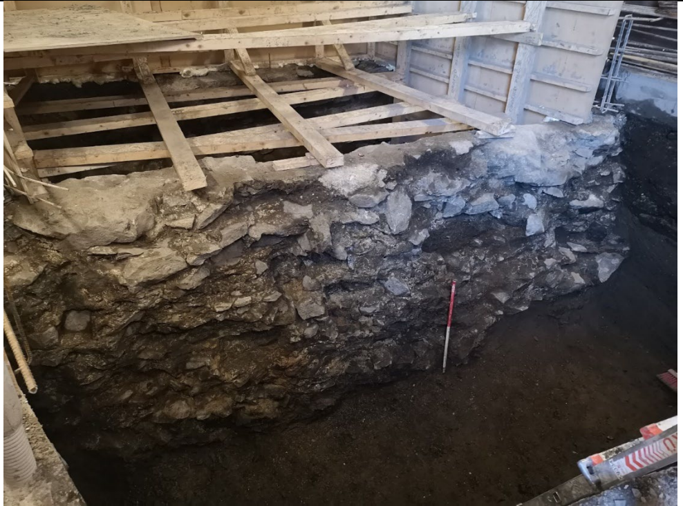
Excavated length of the former sea wall that lies under the Substation
