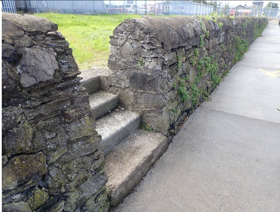
The south parapet of the GSW within the MTL Yard has been breached in several places, in this instance to insert step access
