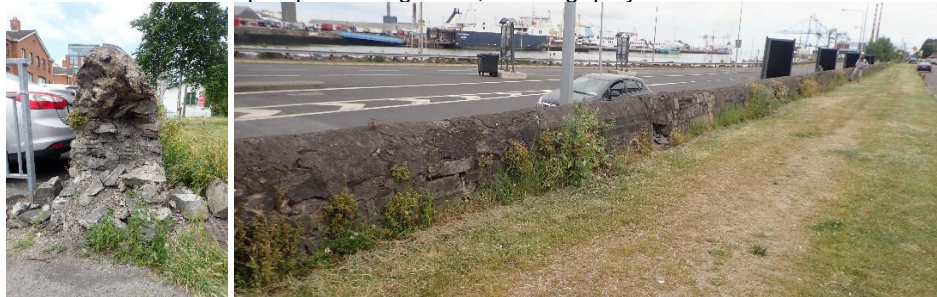
View showing breach in north-facing parapet, and view looking east along north-facing parapet from York Road
