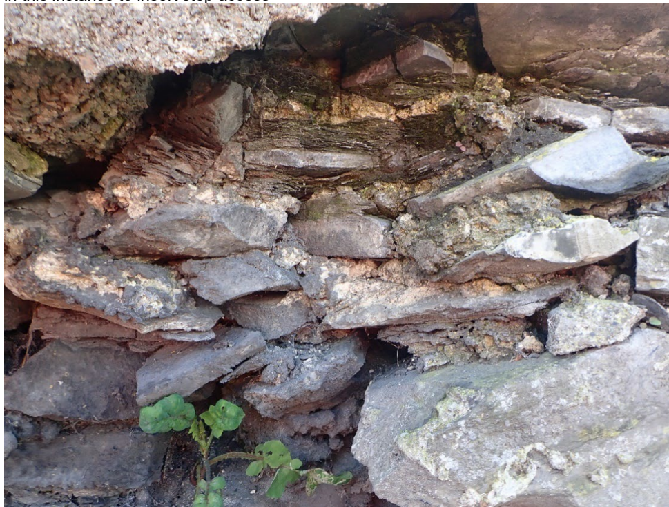
Detail showing fabric of the south parapet of the GSW in the MTL Yard where the wall core is exposed
