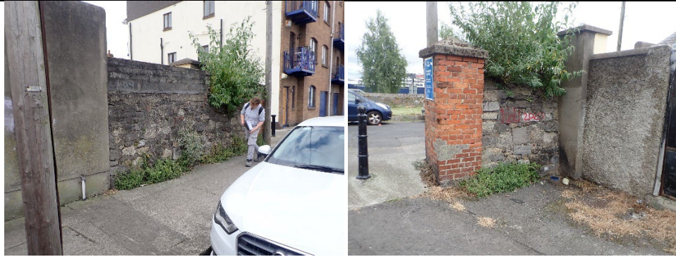
Views of surviving south parapet wall at junction of York Road and Pembroke Cottages
