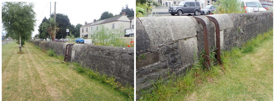
Two views of northern parapet looking south, showing quay wall ladder retained
