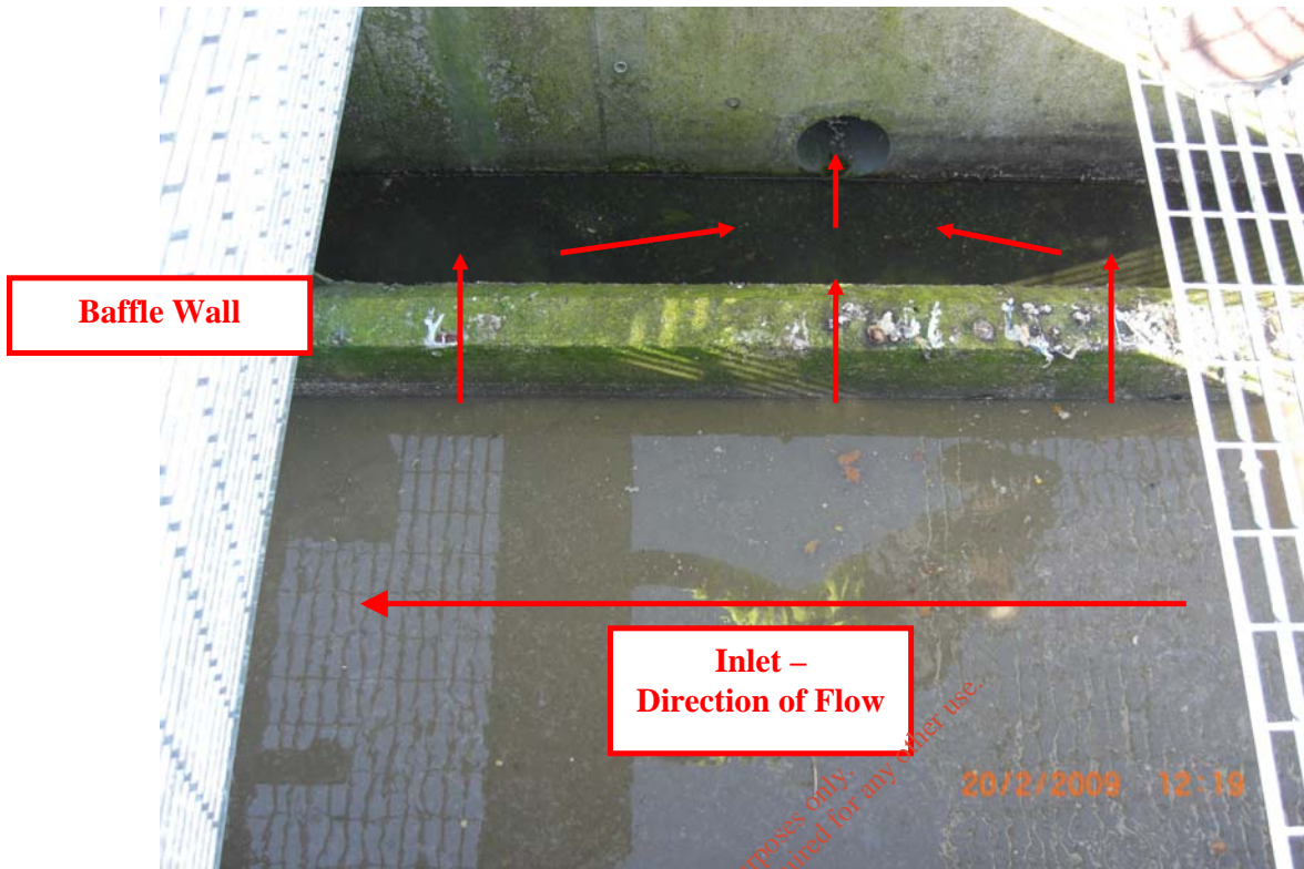
Photo KK-WWDL-207-C.1.1.2 – SWO at Inlet Works in WWTP
