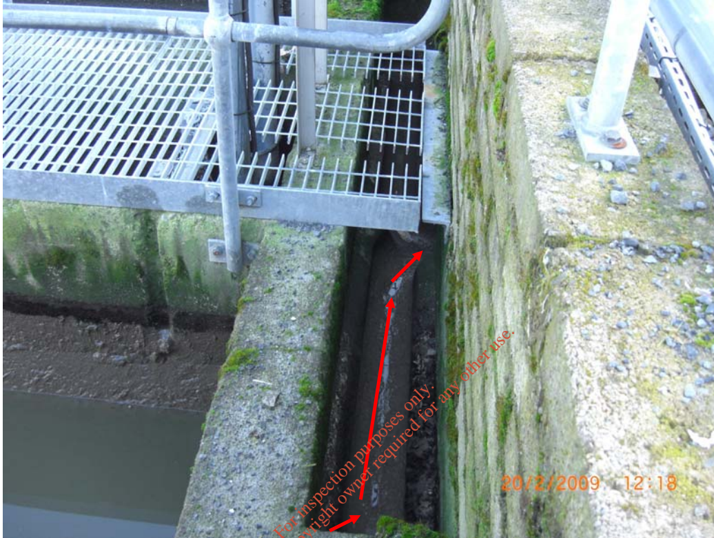
Photo KK-WWDL-207-C.1.1.1 – SWO at Storm Tank in WWTP
