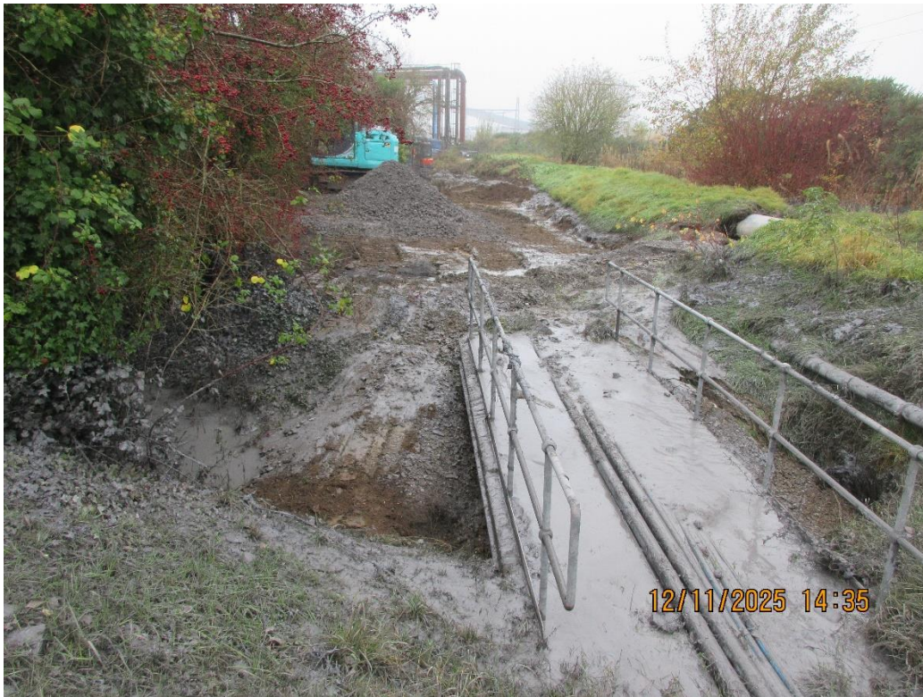
Photograph 1: Tailings in the area around the pipeline failure.
